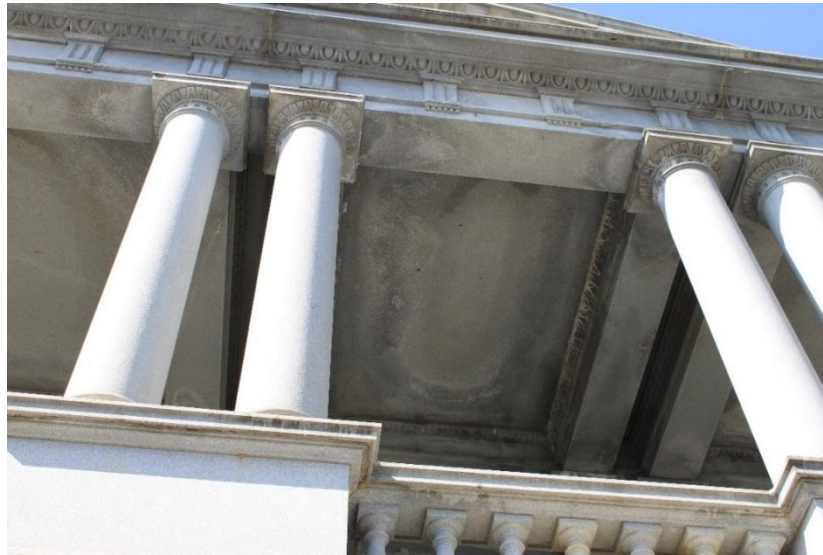
Figure 8: Moisture retention and efflorescence on pavilion ceiling of EEOB, 2026.
