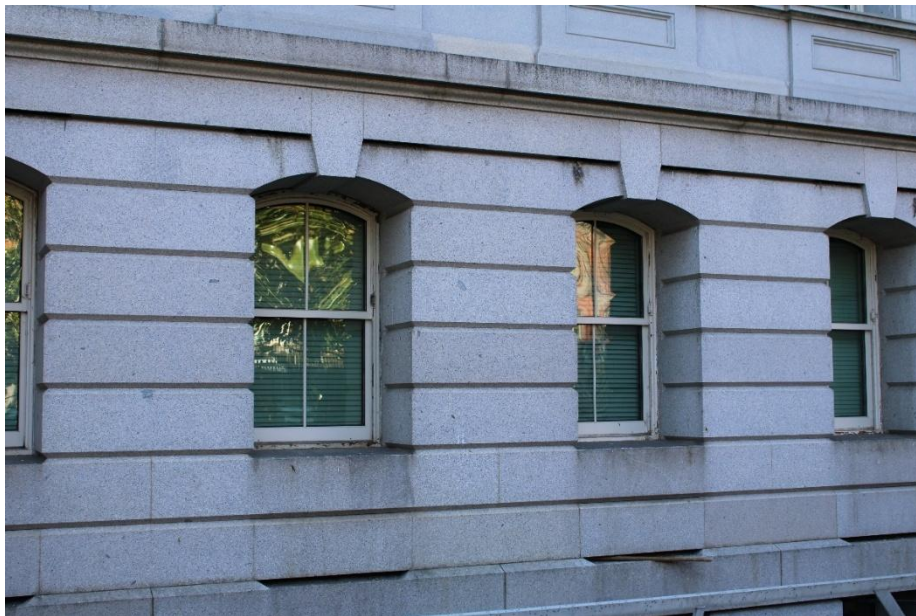
Figure 11: Soiling and bird guano on north elevation of EEOB, 2026.
