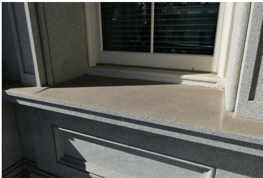
Figure 10: Soiling on granite window sill on east elevation of EEOB, 2026.
